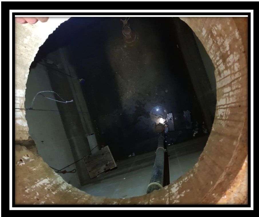
Figure 2A: Sump pump (Tshwane House)
