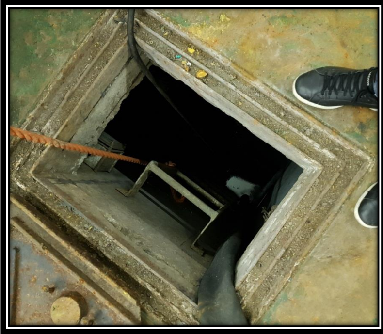
Figure 3A: Sump pump (State Theatre)
