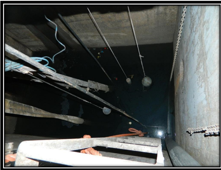
Figure 4A: Main sump pump or pit in the State Theatre
