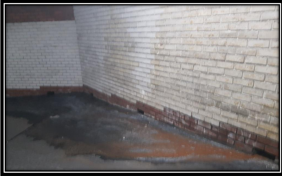
Figure 11A: Wet floor and collecting drain system in Demar Building
