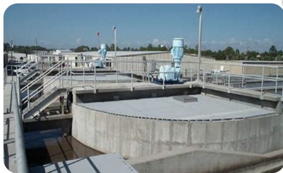
HOMEVALE WATERWASTE TREATMENT WORKS
