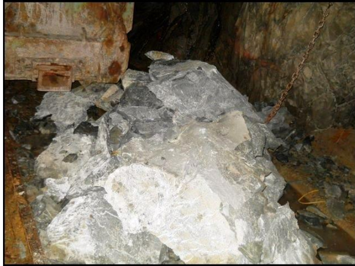
Figure 8-28: 1940 NE E7 X/CUT roof FOG (fall of ground) - 26 July 2011 (provided by BLA Mining Consultants). The FOG was structurally controlled (gravity-induced) and occurred in a highly stressed environment.
