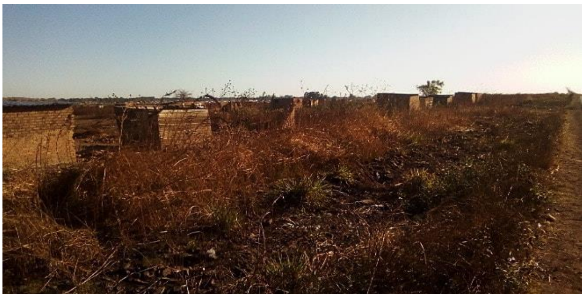
Plate 8.1: Illegal housing structures re-erected at Arlington Estate by former members of Nyikavanhu Housing Cooperative after demolition in 2016
