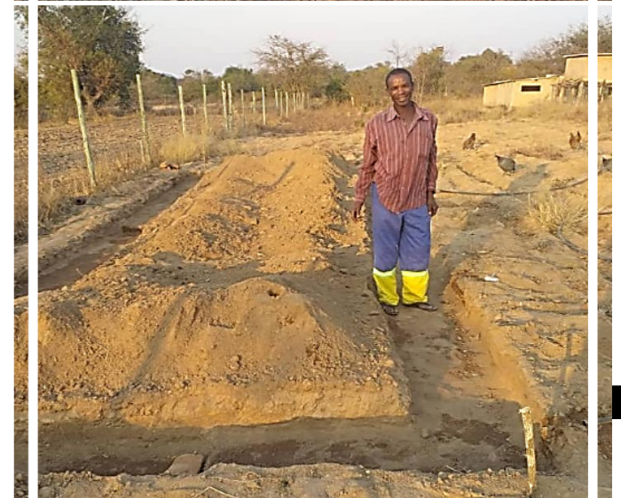
Figure 24: Collage of the local clay bricks and shallow raft foundations for communal house construction (Author, 2020)
