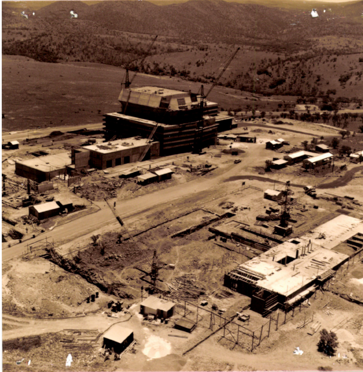
Figure 16: Pelindaba under construction, with the main housing for the SAFARI-1 reactor visible as built structure (NECSA, n.d.).
