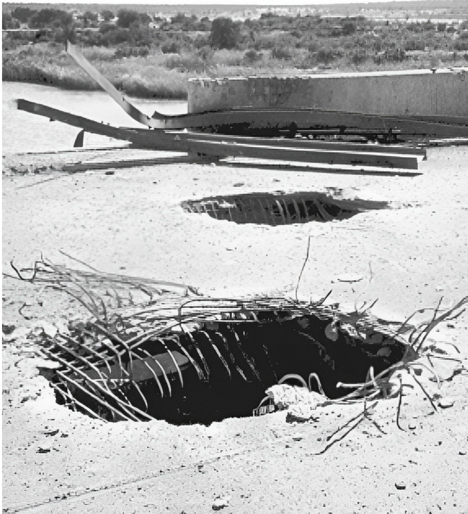
Figure 12: Bombed out structures of the border (Venter, 2019).
