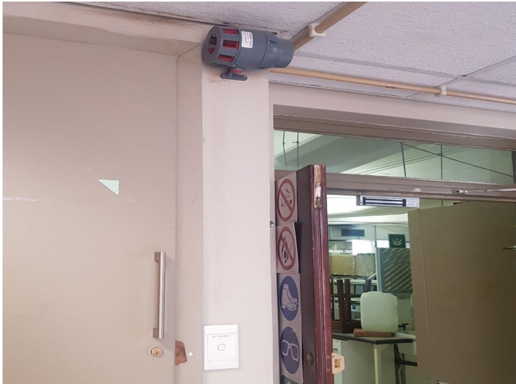
Figure 4.10 Alarm siren near the door at the chemical lab
