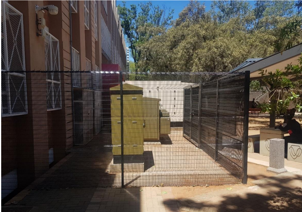
Figure 4.12 Barricaded electrical transformers
