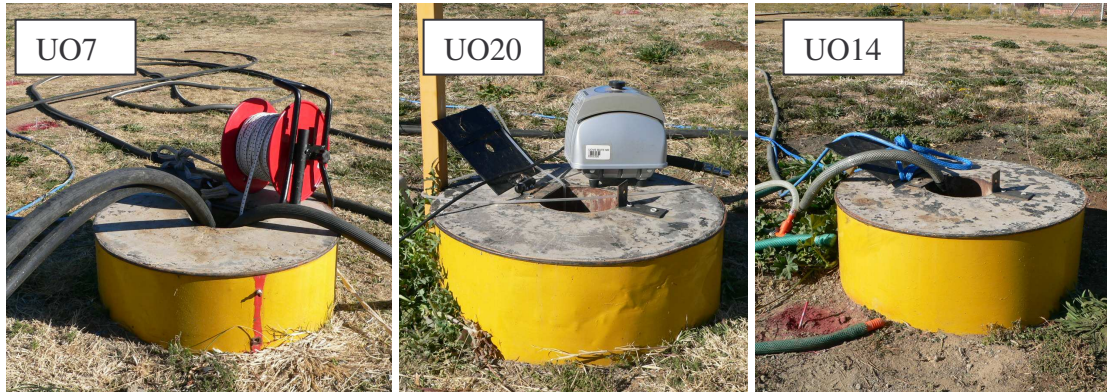
Figure 6-1 Set-up of the three boreholes: UO7 (injection borehole), UO20 (observation borehole) and UO14 (abstraction borehole).
