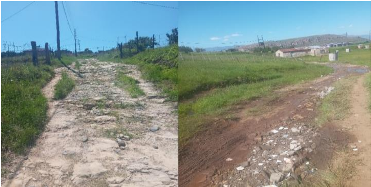
Figure 41: Poor Roads in Makwane and Matsikeng (Fieldwork Images, 2023).
