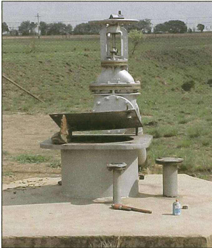
Figure 3-3. Example of a remaining borehole casing at Minnaar Colliery.
