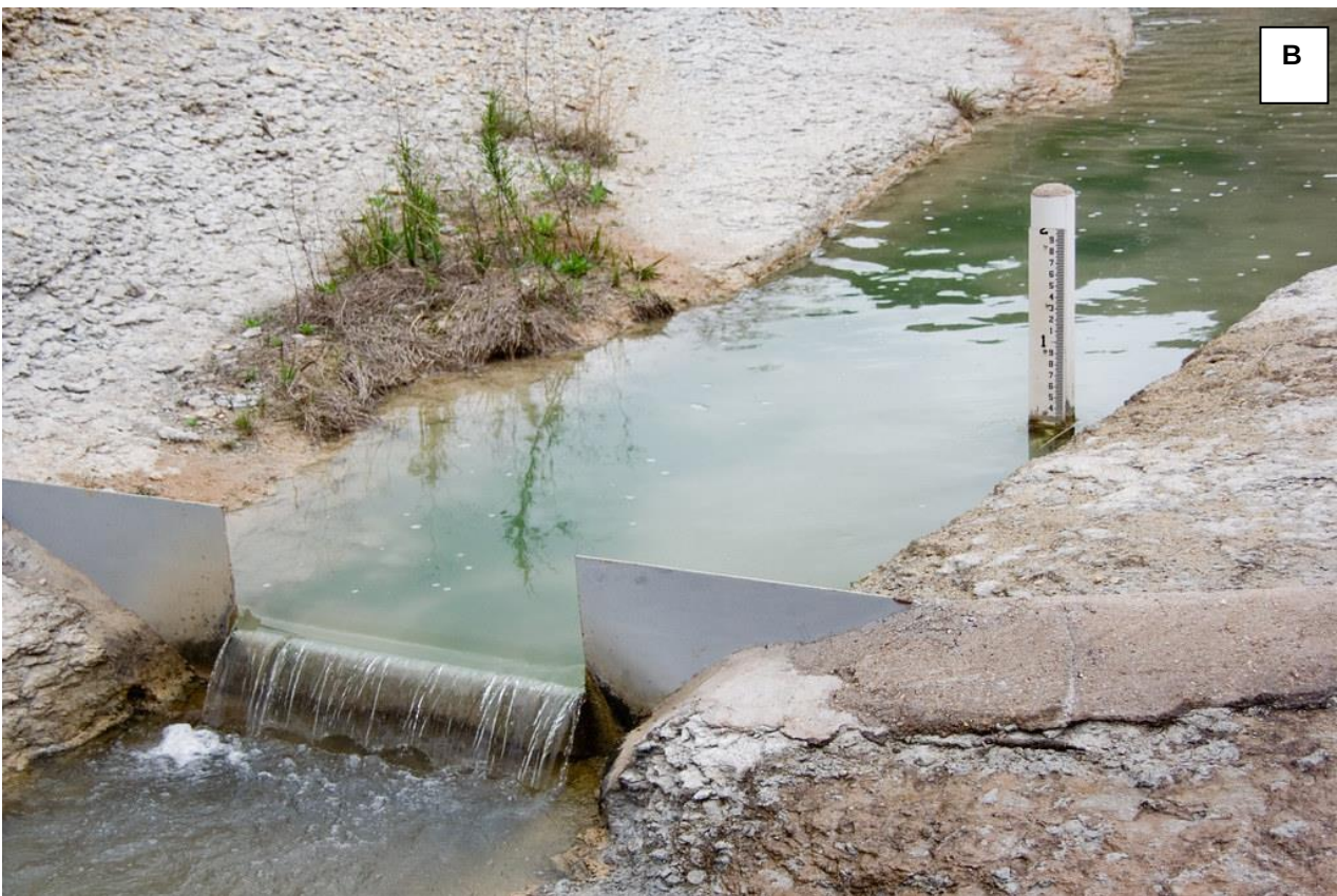
Figure 3-4: Example of a rectangular weir similar to the rectangular weir installed at the outlets of the Lower and Upper Fountain Springs (Modified from Loughborough University, 2023 and Emito, 2023)
