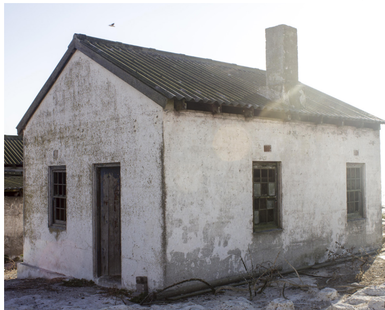
Fig 2,113 Nature has clearly had an effect on the existing structures
