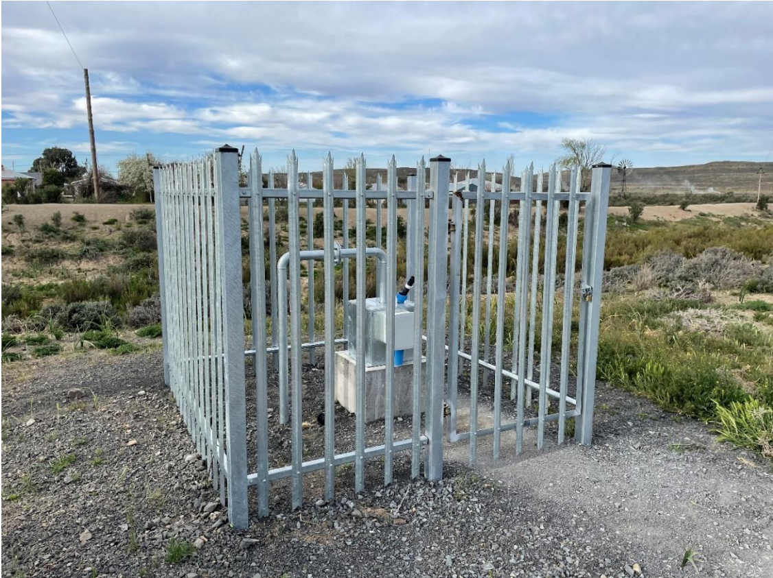
Figure 1: Example of a protected production borehole with enclosure and proper monitoring infrastructure
