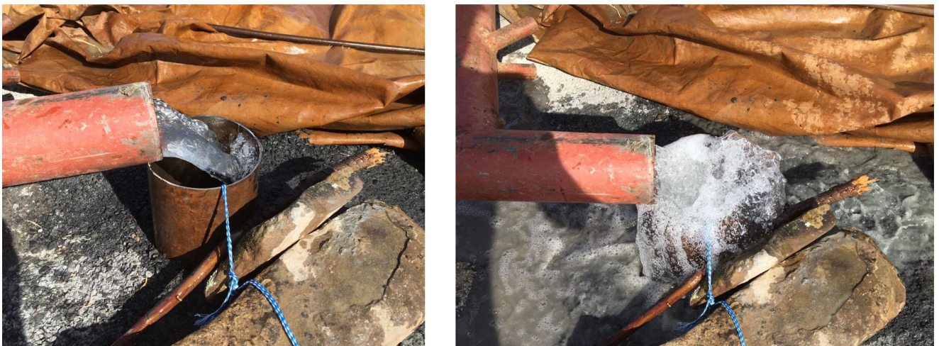
Figure 67: Photographs of the modified falling head test conducted on borehole MAR2, injection (left) to overflow (right) (author's own)
