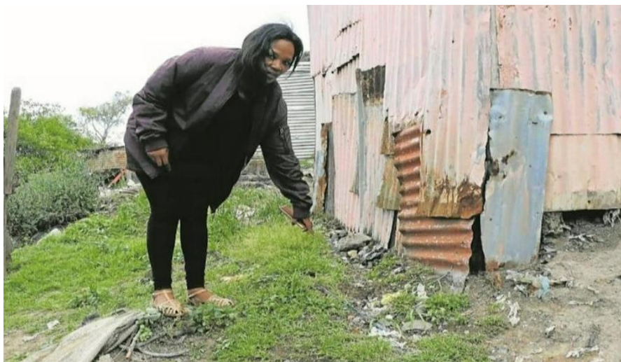
Figure 2.5: Niece of the late woman showing where her aunty was electrocuted by illegal electricity
