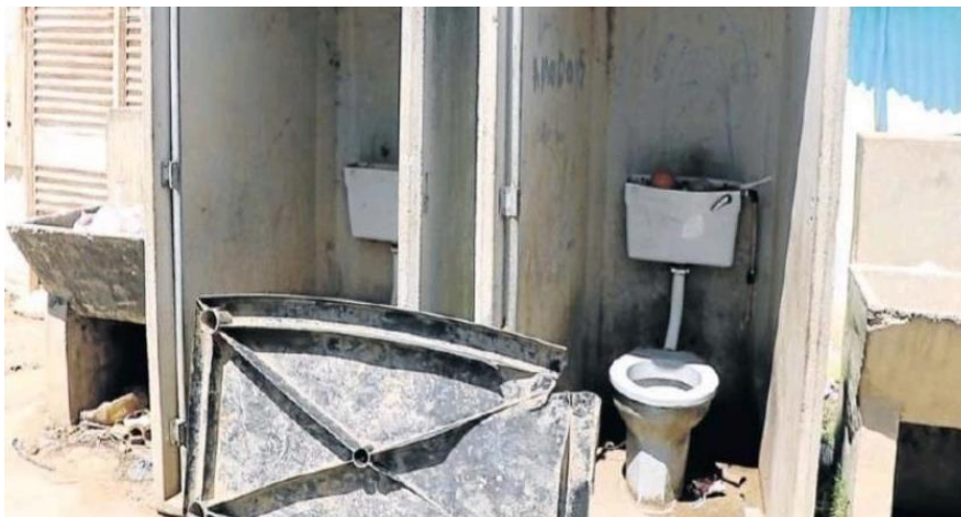
Figure 2.4: Dilapidated toilets at the Nompumelelo informal settlement
