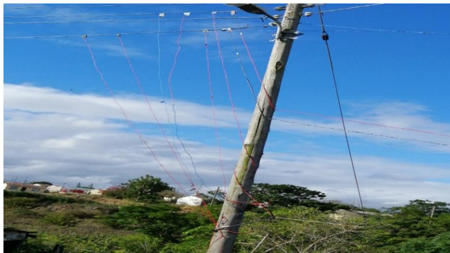
Figure 6.8: Illegal connection of electricity in one of Mdantsane informal settlements
