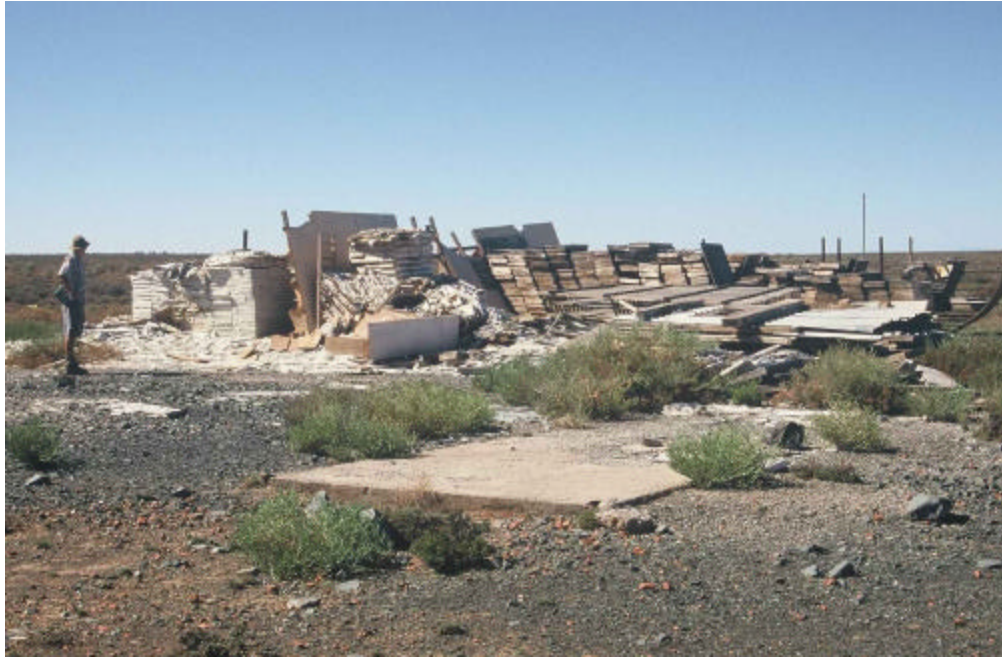
Figure 3.1.5 Collapsed core sample storage on Ryst Kuil (no. 1 on location map).
