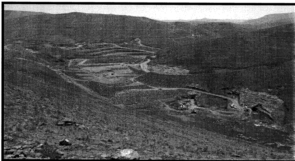
Figure 4.6-2: Mohale Gorge: Construction of the Dam at its early Stage. Diversion Tunnels. Dam Embankment. Further Upstream is Quarry for Rockfill Material. Photograph was taken looking Upstream from Engineers Office.
