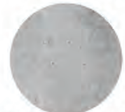
Polished concrete floors
