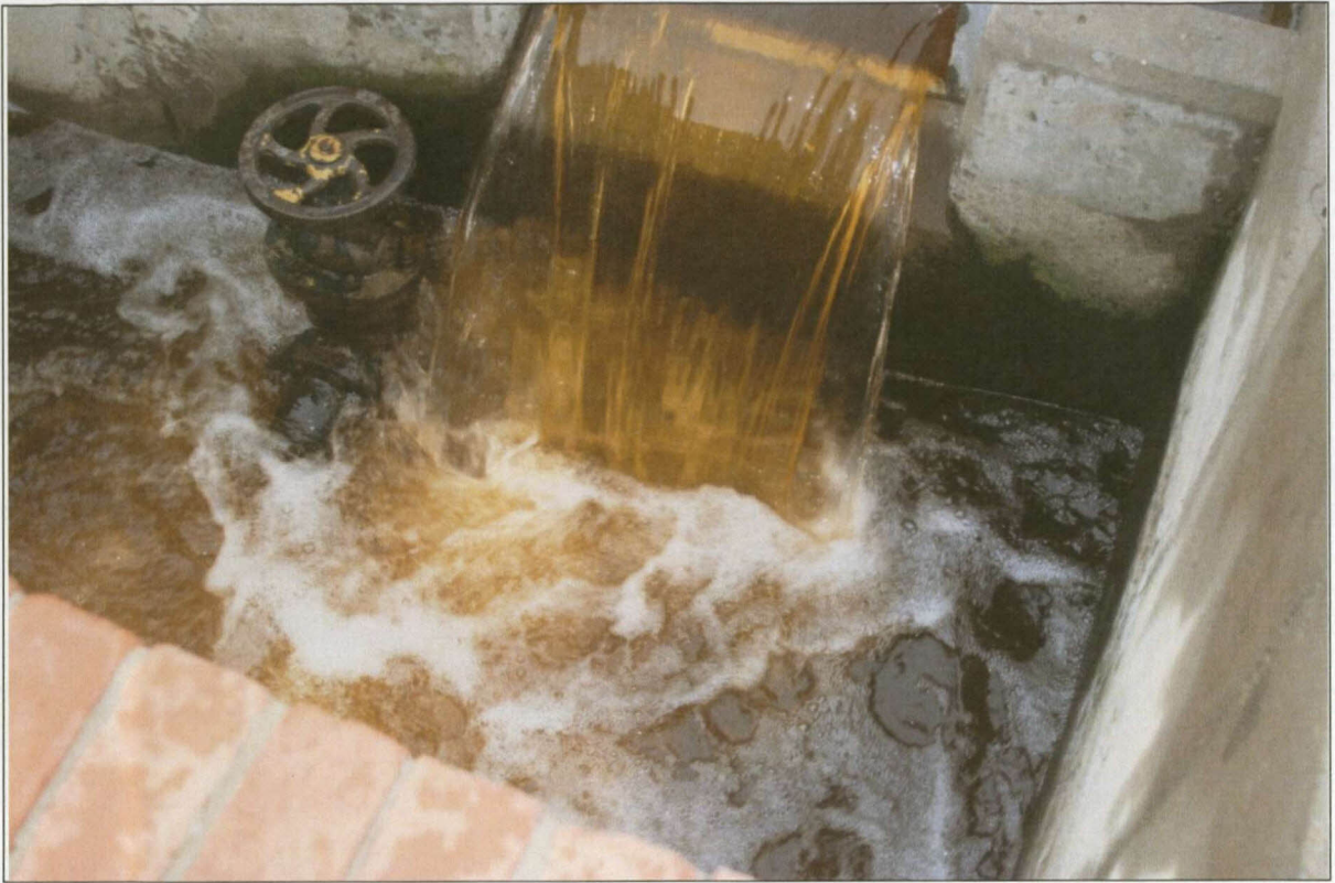
Figure 5.16: The red-brown coloured sewage effluent at the exit point from the Thaba-Nchu sewage treatment plant (Photo taken: August 2012)
