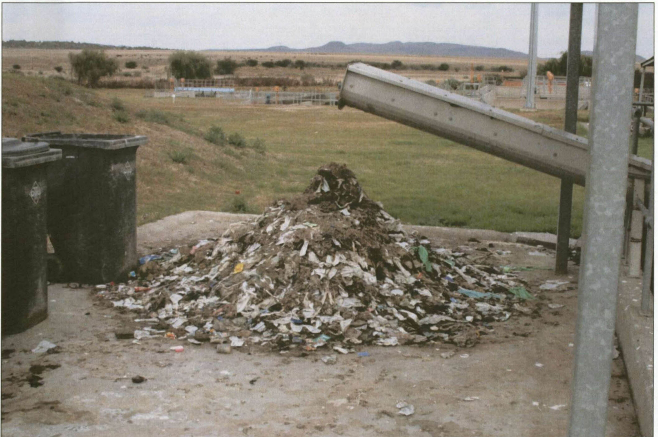
Figure 4.15: Screening process at Thaba-Nchu WWTP (Picture taken: August 2011)
