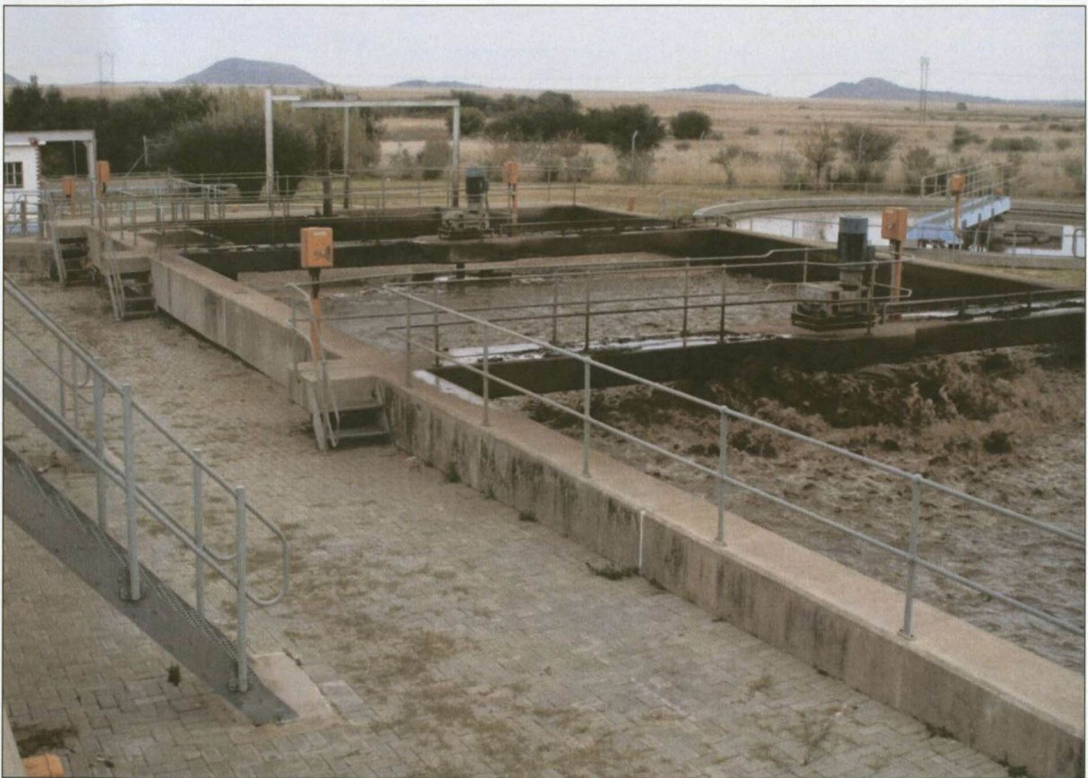
Figure 4.19: Mixer tanks at Thaba-Nchu WWTP (Picture taken: August 2011)
