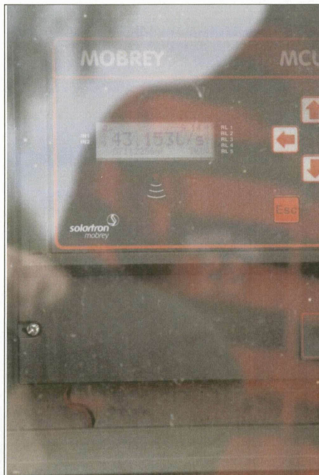
Figure 4.17: The effluent flow meter displaying an incorrect figure of 43 153 l/s (Picture taken: September 2011)
