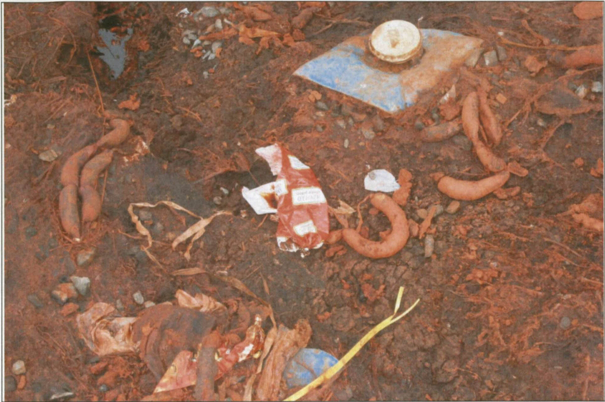
Figure 5.15: The details of the factory waste and the manhole through which factory waste joined the sewage stream for treatment (Picture taken: June 2012)
