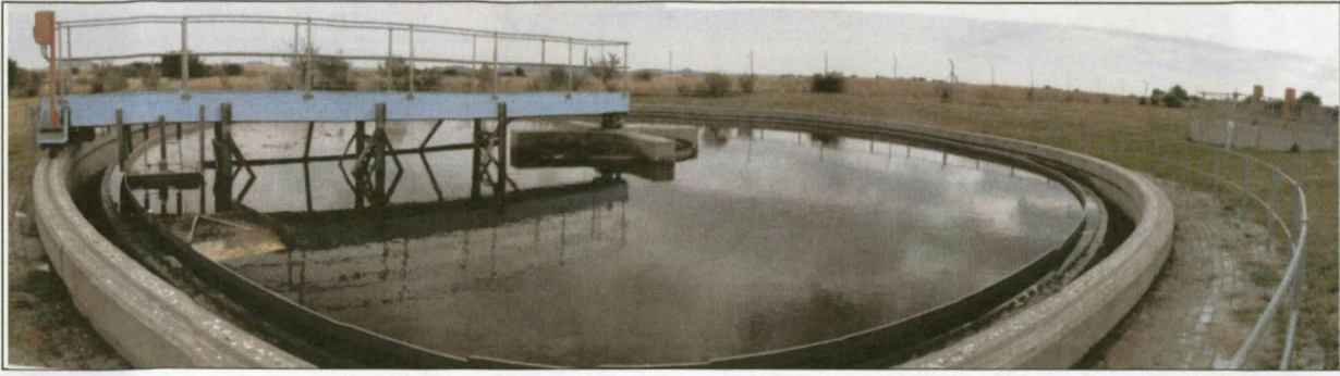
Figure 4.21: A final settling tank at Thaba-Nchu WWTP (Picture taken: August 2011)
