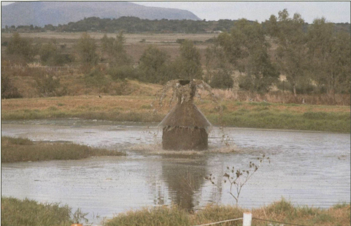
Figure 5.4: The working aerator at the sewage treatment plant (Picture taken: April 2012)
