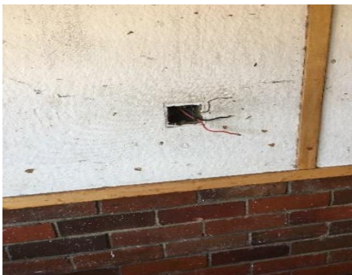
Figure 4.5: Vandalized power outlet in one of the lecture rooms
