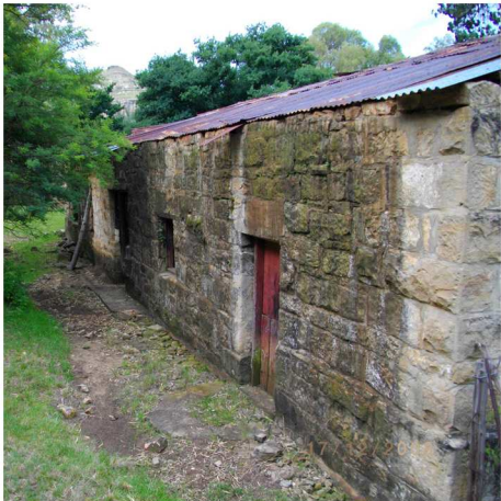
Fig. 154 Western side of house with back door in front and front door behind, in the shade. (Photo: Louis du Preez 2012)
