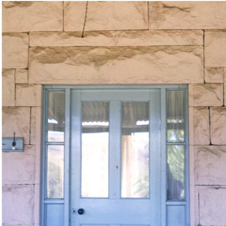
Fig. 240 Front door, showing detail of lintel and adjustment to courses of the wall. (1987)
