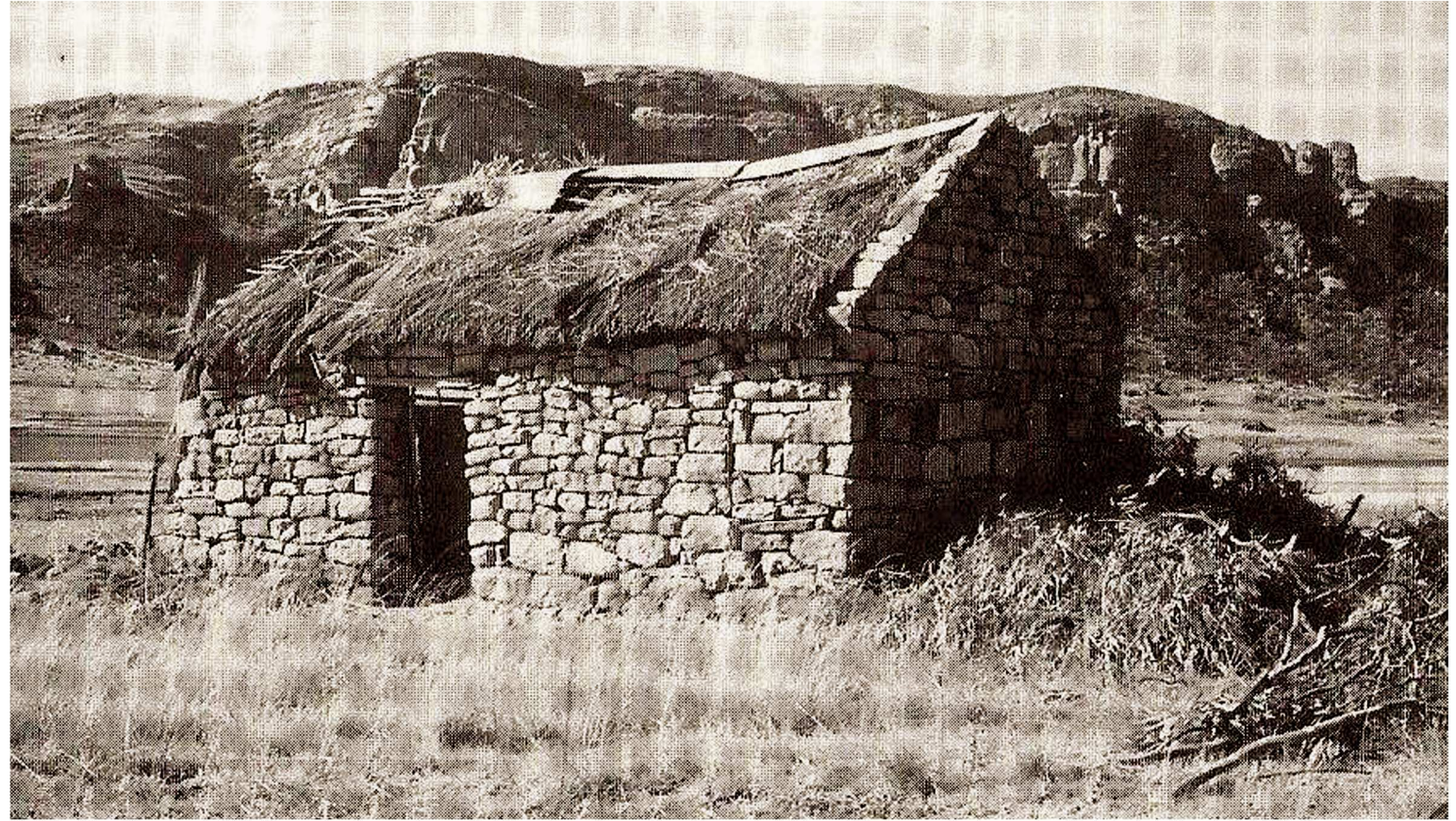
Fig. 9 Condition of the cottage in 1979. The remains of a parapet were still visible on the southern gable and the wooden lintel was still in place over the door opening. (Photo: Louis du Preez in Eloff 1980: 5)
