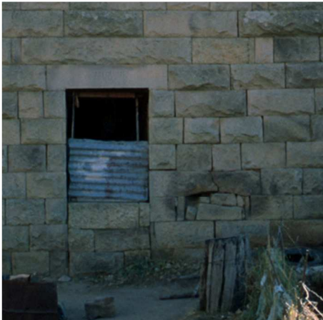
Fig. 60 Detail of door turned window with inscription above it and oven hole next to it. Note huge second lintel above lintel. (1999)
