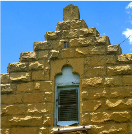
Fig. 39 Detail of step-gable on north-western side of house with trefoil arch over loft door. (1987)
