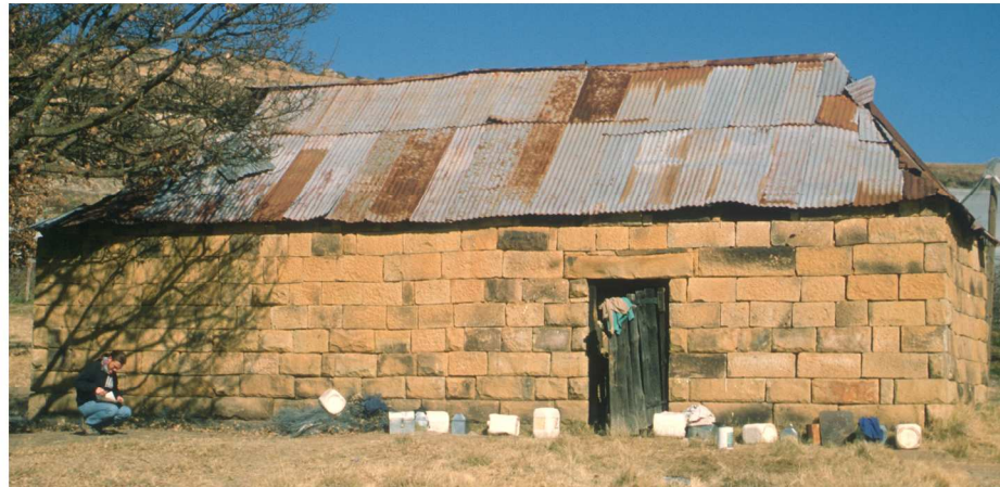
Fig. 64 Shed on northern side of house. Stonework display influences of both the house (rockfaced sandstone) and the rondavel (rough hammer-dressed sandstone) on the same structure. (1999)
