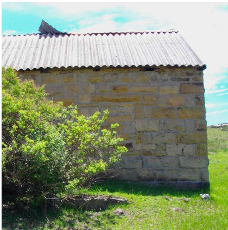
Fig. 191 Southern corner seen from the western side with remnants of steep in front. (Photo: Louis du Preez 2012)
