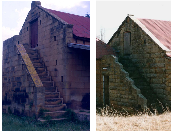
Fig. 295 & 296 The stonework at Tierhoek (left) (1987) is precise and ordered like the plan. The stonework at Schoonzicht (right) (1999) includes unusual refinements like the chisel drafted margins and the large interlocking stones on the handrail of the staircase. In spite of these refinements, the stonework on Schoonzicht was not done neatly. All sorts of inaccuracies were ignored by the builder and was absorbed in the larger whole. The plan introduced a new form (the double bank plan) to this collection of houses in the Basin, but are remarkably careless in placing doors at strategic points.
