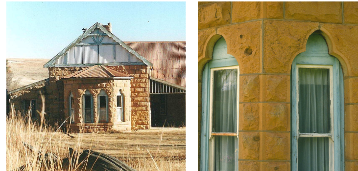
Fig. 307 & 308: The bay window (left) on the south-eastern side of Dunelm (1999) with a detail (right) of the stonework and woodwork involved. (1987)
