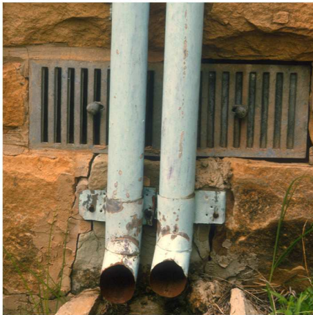
Fig. 58 Detail of double downpipes and sub-floor vent grilles on north-western bay window (1987)
