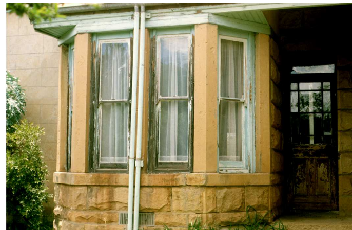
Fig. 43 Bay window on north-western side of house with double downpipes and double sub-floor vent grilles behind the downpipes. (1987)
