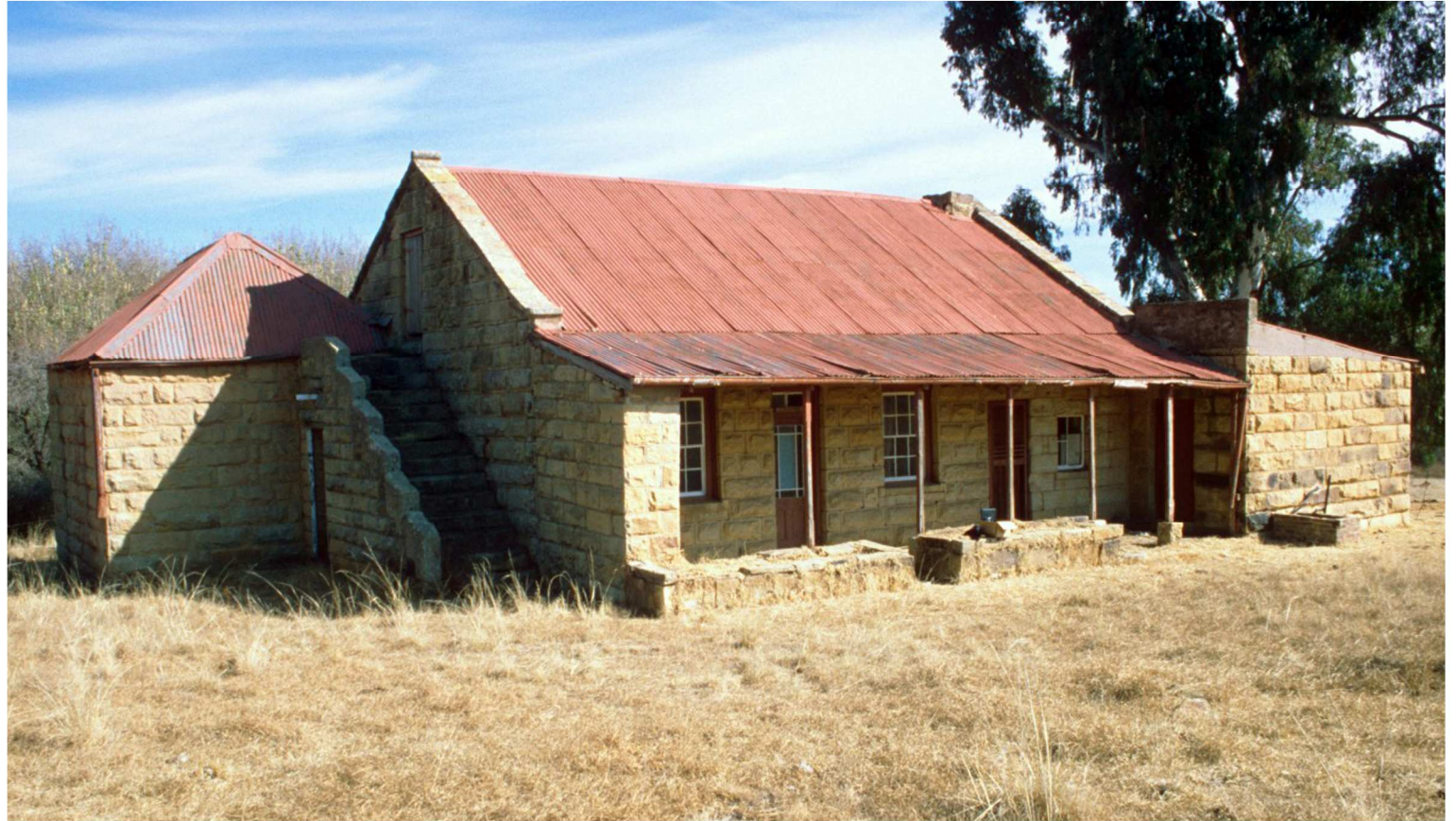
Fig. 201 Eastern elevation showing back stoep and doors to living/dining room (left), kitchen (centre) and bathroom (right). (1999)
