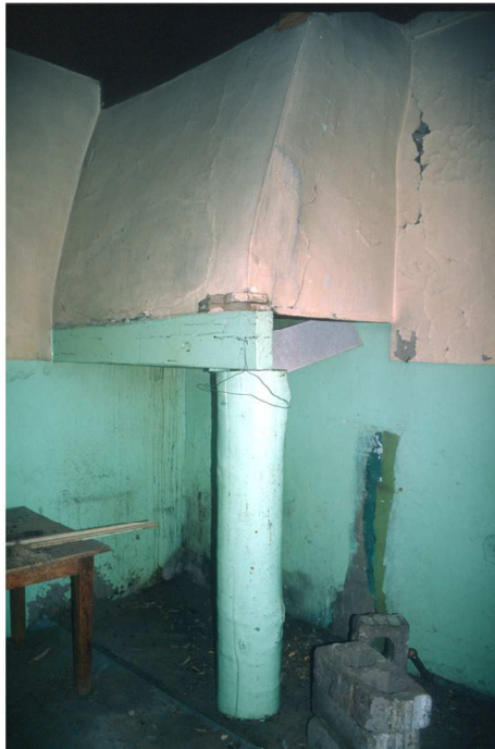
Fig. 208 Hearth in the kitchen of Schoonzicht with masonry hood supported on timber post. (1999)
