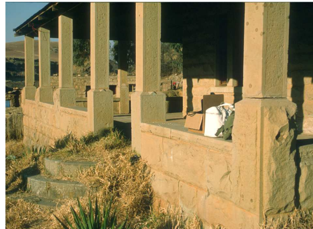
Fig. 76 Corner of stoep showing the columns of the new stoep. Note also the differences in detailing on columns. The corner column and base are different from a column in the middle of the row or from a column next to the entrance. (1999)
