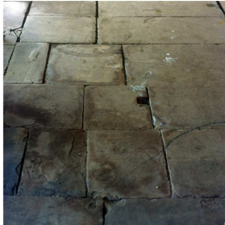
Fig. 252 Original flagstones of sandstone on the 1899 stoep, shown here polished with ordinary floor polish. Sandstone flagstones were used extensively in the Brandwater Basin, for instance at the school buildings. It was not a successful paving material in the long term and most of these surfaces were replaced with an alternative material long since. (1987)
