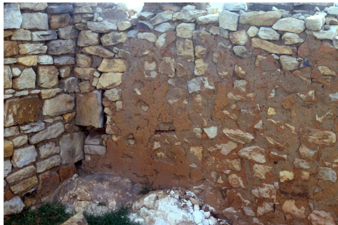
Fig. 19 The south-western inside corner showing the boulders that have always been inside the cottage. Note also the different building techniques: on the wall (right) and gable on left. (1987)
