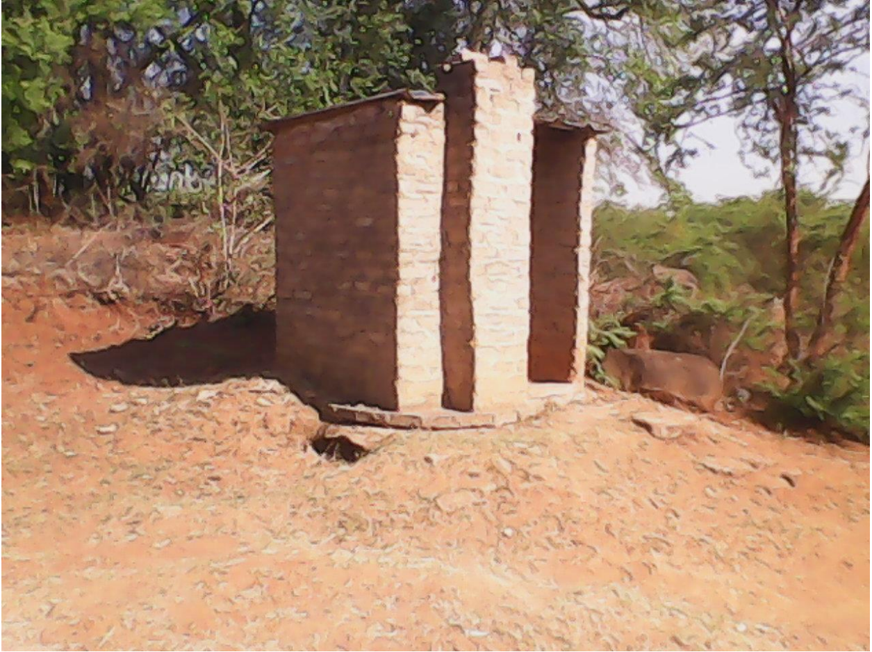
Plate 4.9: Insufficient and risk toilet for farmers and insensitive to gender (Rozva)
