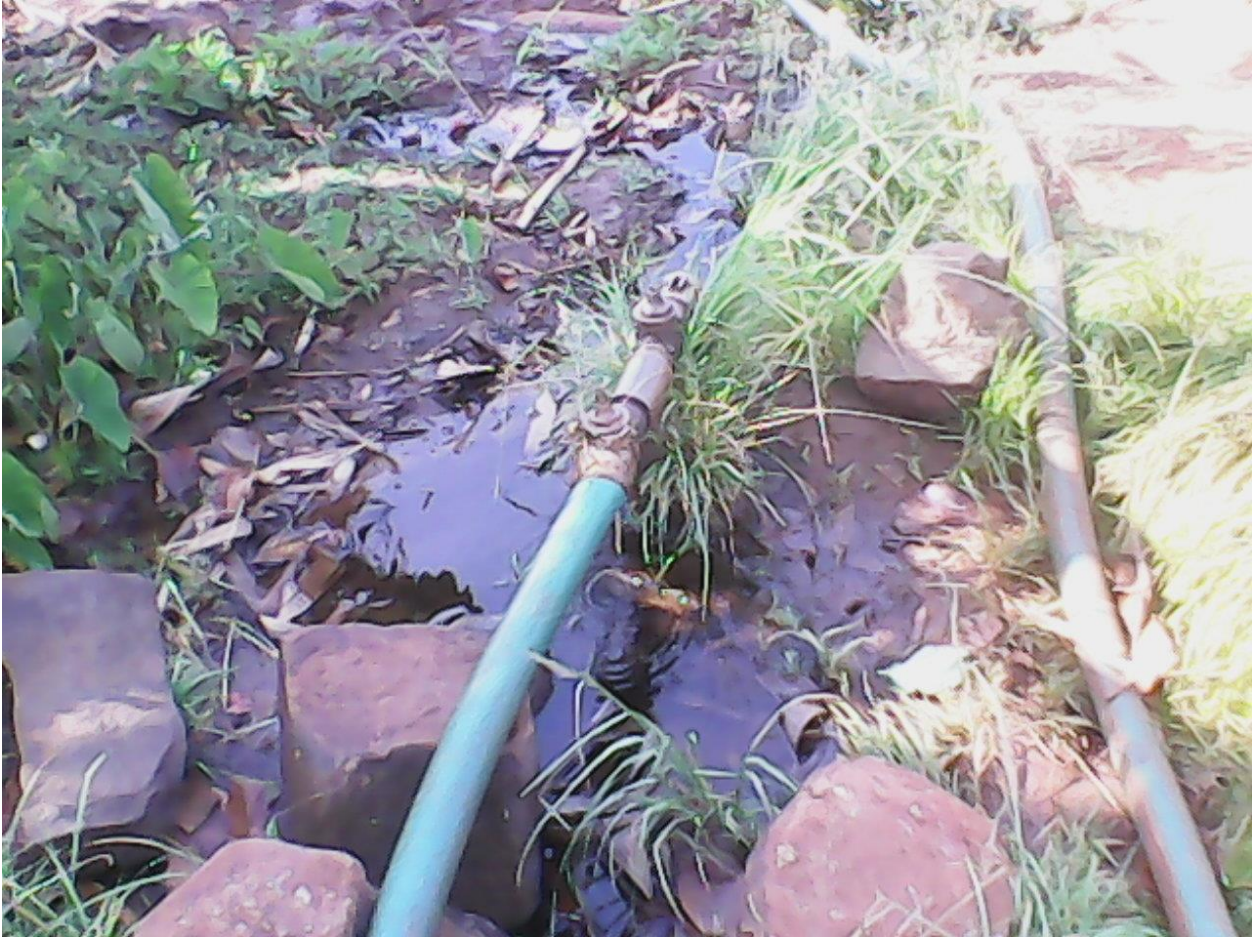
Plate 4.4: Poorly maintained broken and leaking pipes (Rozva)
