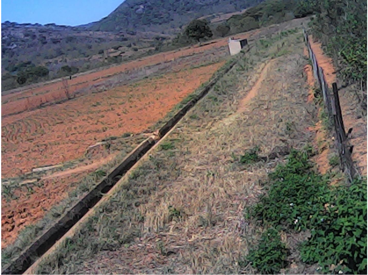
Plate 4.3: Subserviced canals with cracks and weeds growing inside (Shereni)
