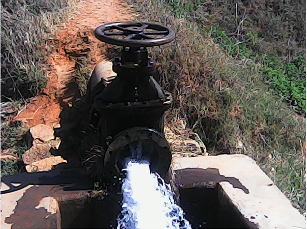
Plates 4.2 : Poorly maintained, unprotected and exposed hydrants (Shereni)
