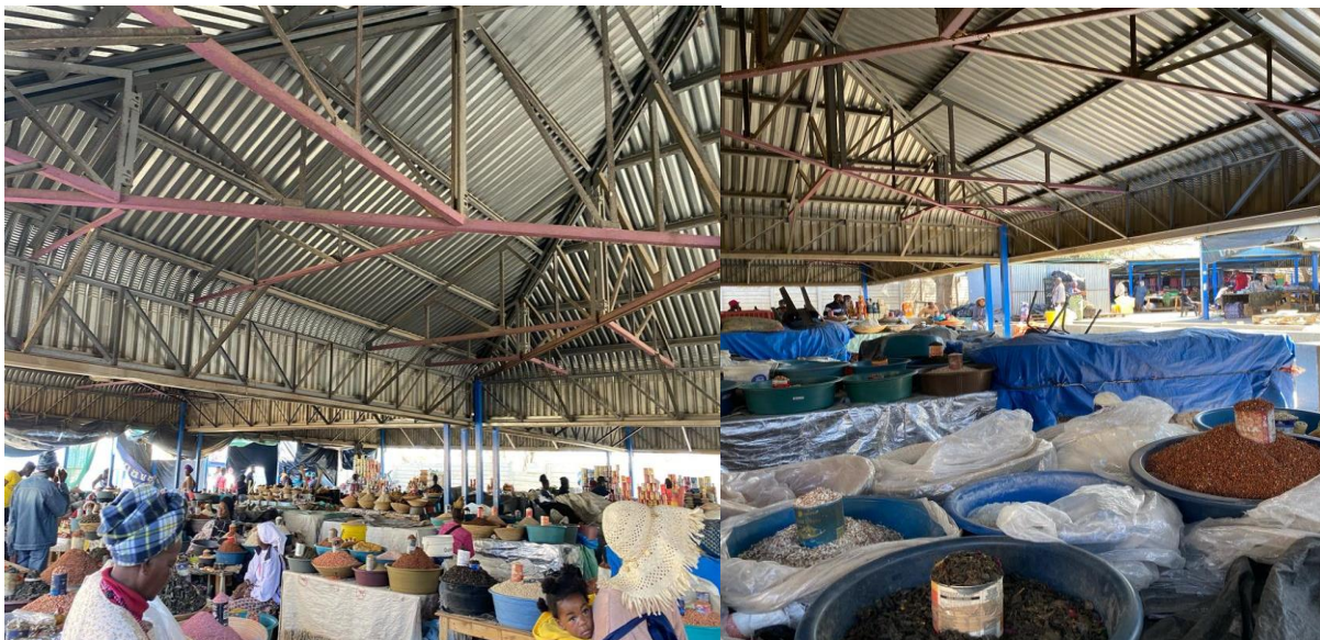
Picture 6.3.3: The Tukonjeni Informal Market Structures Also known as the “Stop ‘N Shop Informal open market, 2023.
