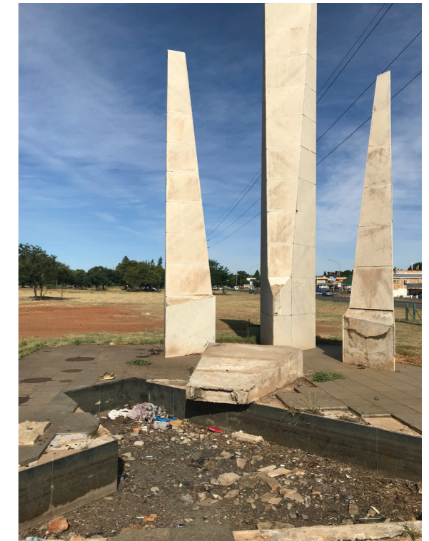
Figure 4.54 Urban decay (Author, 2018)
