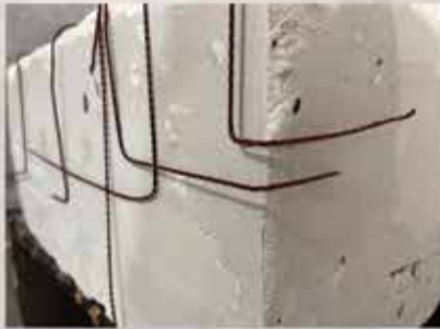
Figure 187, Twisted wire wrapping around base, (author)
