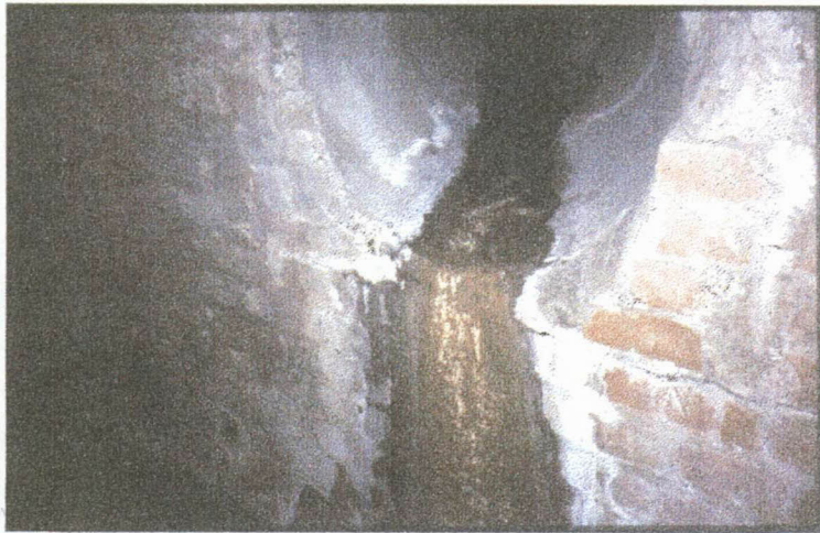
Photo 7: A waste pipe leaking into the canal.
