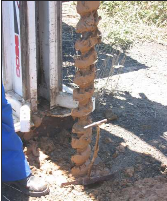
Figure 7-2: Caking of sand and clay slurry during auger drilling.
