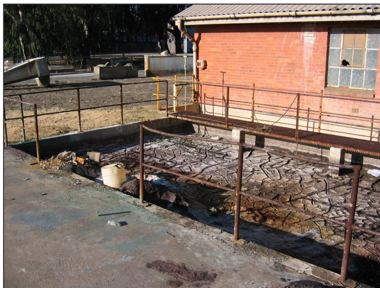
Figure 6-12: Lime treating and wastewater holding facility.
