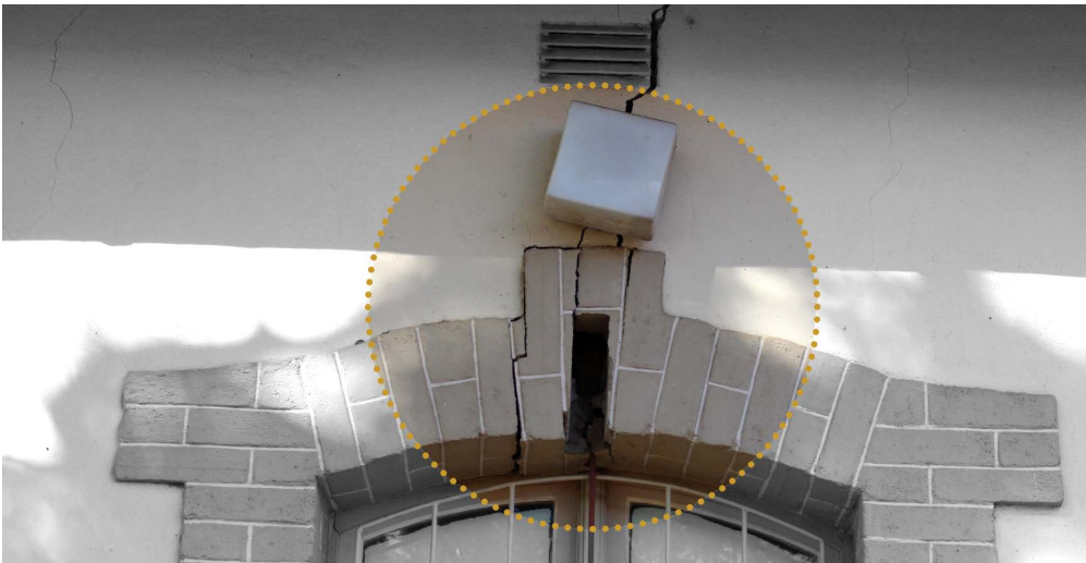
Fig. 24 Structure shows deep cracks possible due to differential subsoil settlement. Structural integrity will have to be investigated in this regard. Photograph: Author, 2018.
