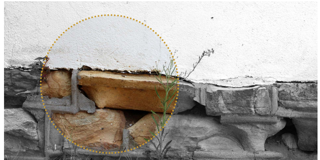
Fig. 21 Clay foundation walls and plinth in overall poor condition due to decay and weathering which can possibly undermine the structural integrity of the building. Photograph: Author, 2018.
