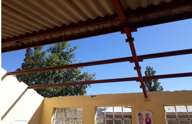
Figure 4.3 Leaking classroom roof and broken windows in School B, showing a non-conducive learning environment
