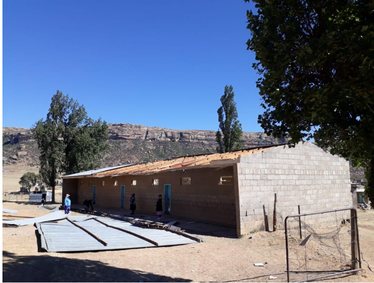
Figure 4.1 Classroom roof blown away by the wind in School A, showing inadequate infrastructure
