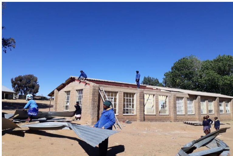
Figure 4.2 Classrooms without ramps; their roof was blown away by the wind in School A, displaying a non-enabling environment
