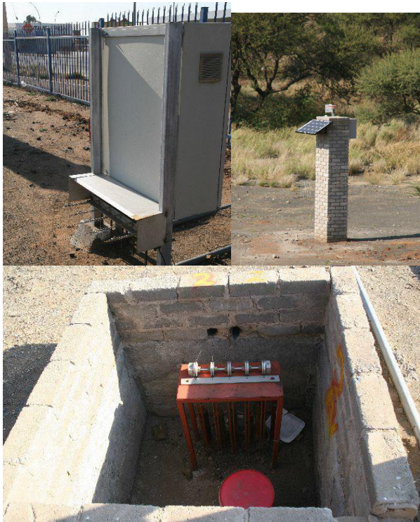
Figure 169: Geotechnical Monitoring Systems (Maree,2017)
