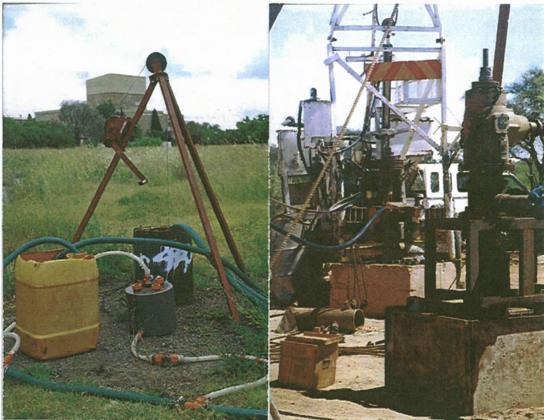
Figure 5-2 Equipment installing at injection and abstraction borehole; a) submersible pumps with a flow rate of 0.3 to 1 L/s, b) mono pump rigs, discharging up to 20 L/s
