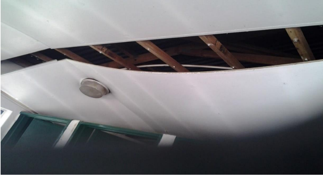
Figure 4.8: Ceilings about to fall
