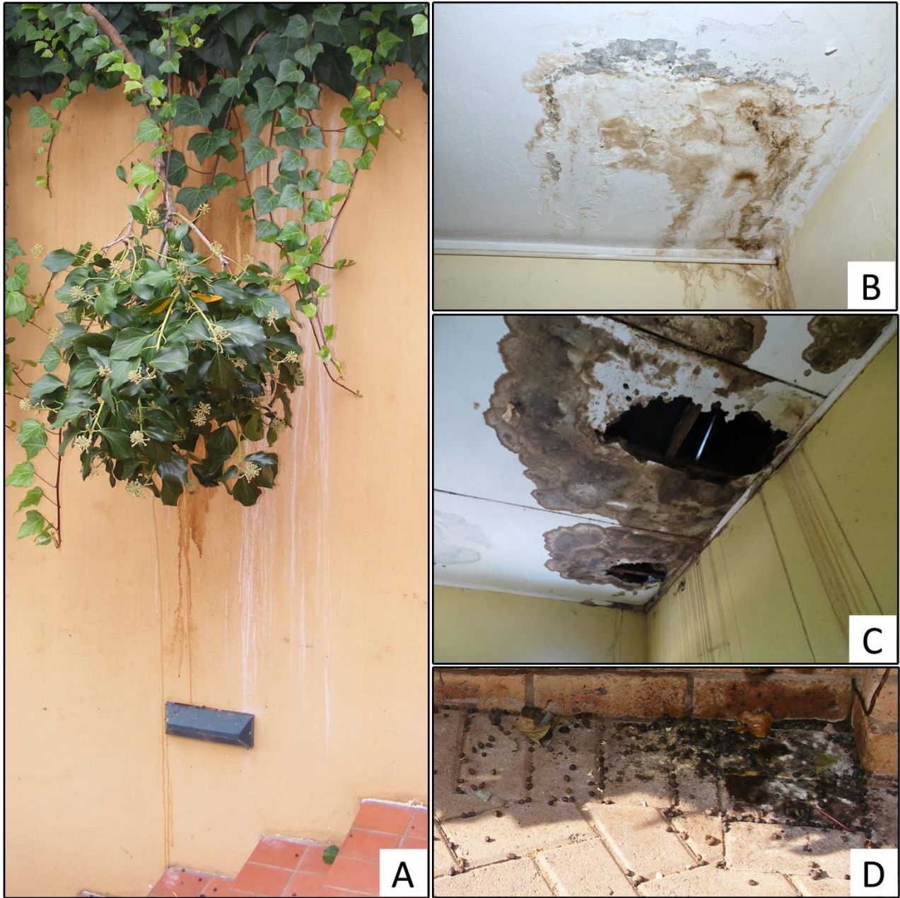
Figure 4.7 Damage caused to structures by hyrax middens included stains to walls (A), damp ceilings (B), collapsed ceilings (C) and stained paving stones (D).
