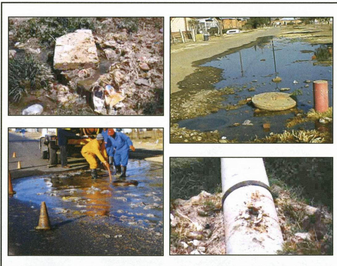
Photograph 6.3 Blocked and vandalised sewer pipes in the study area.
