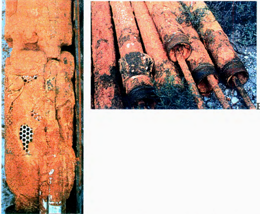
A represents the clogged pump-inlet of DP28 and B the clogged rising main of private borehole VG2
