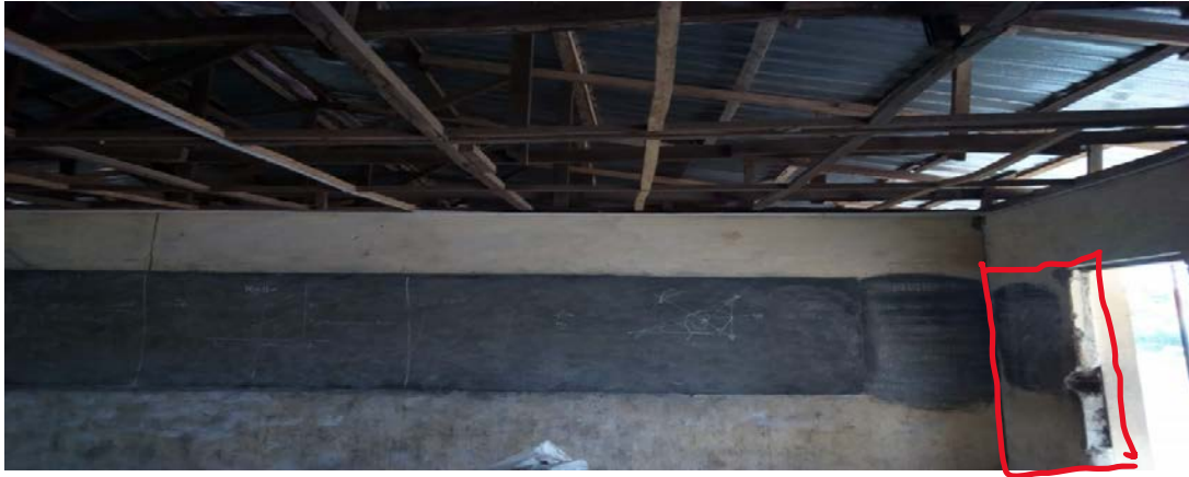
Figure 5.20: Unsafe learning environment (no classroom door, no ceiling, nor asbestos, direct heat, only roofing sheets)
