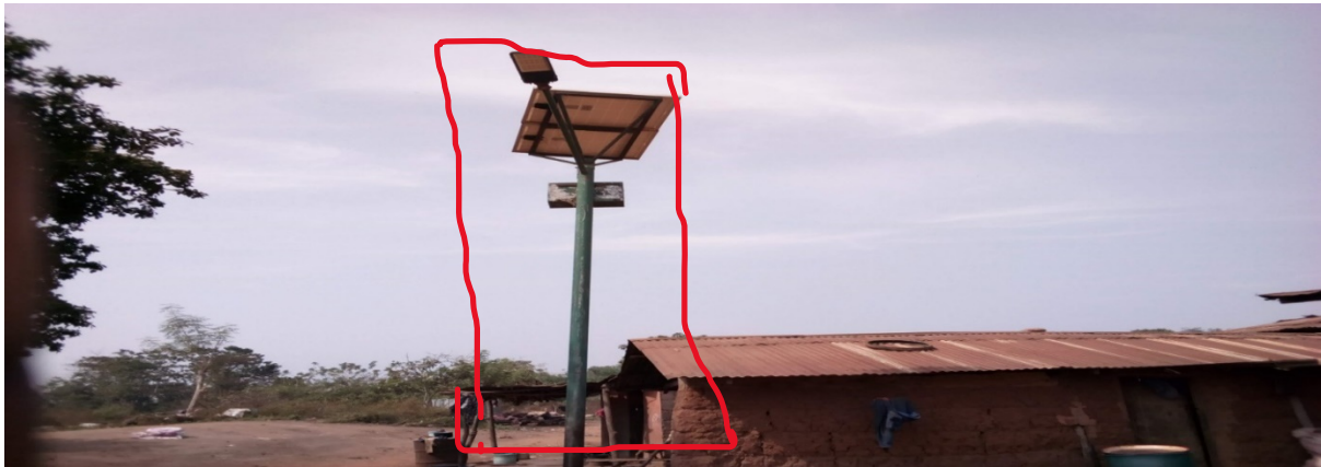
Figure 5.25: Rural electrification powered by solar energy
