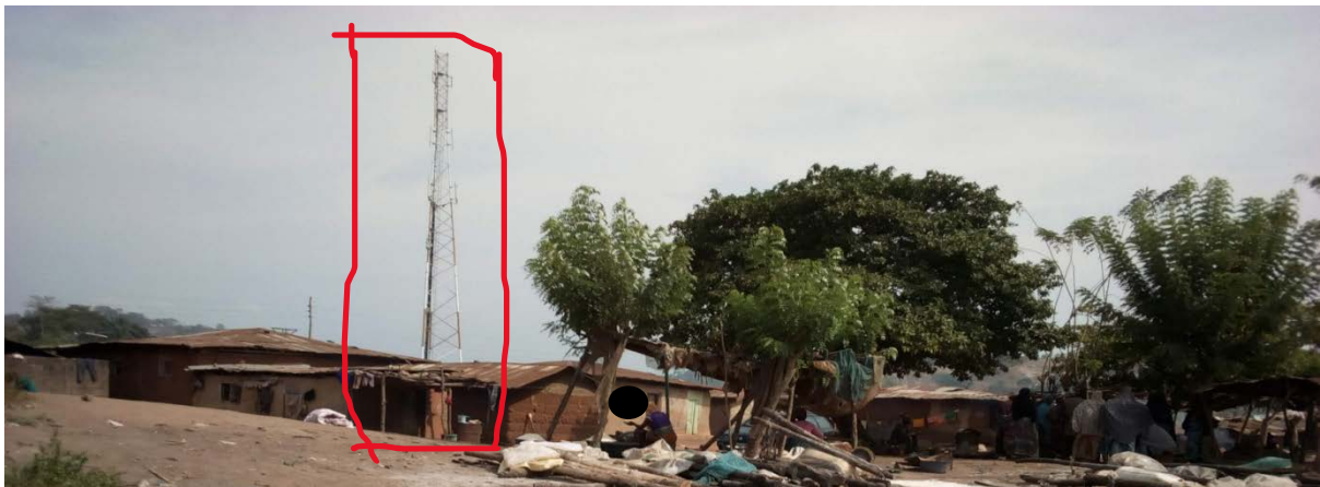
Figure 5.26: Telecommunication mast for mobile phone users in the rural environment
