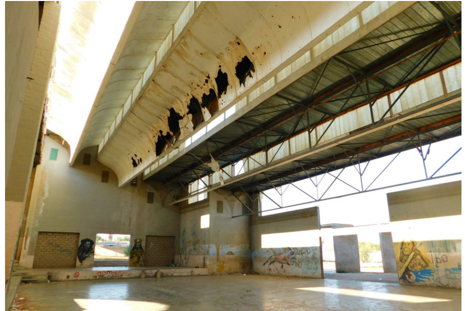
Figure 185: The interior perspective of the building show the disintegration of the ceilings (author, 2022).
