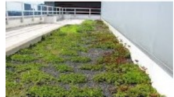
Figure 167: Use of green roofs. (Phun, X. Y. 2012: 2)
