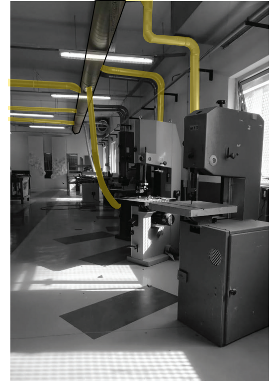
Figure 33 Workshop ventilation system(Saunders. 2019).
