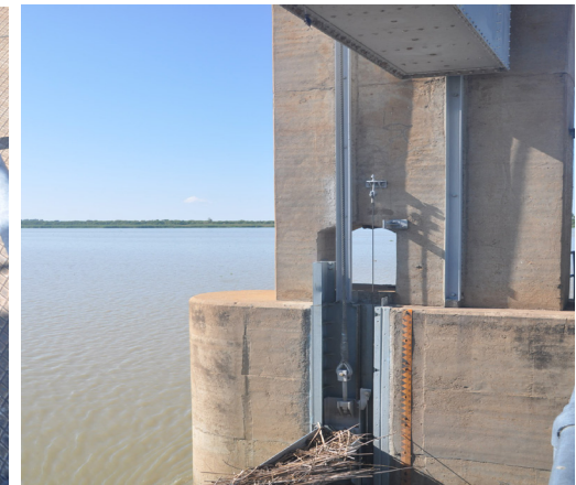
FIGURE 18: The system control connections to the sluice (Author, 2023).
