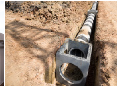
FIGURE 352: Storm pipe (GSM plumbing, 2021).
