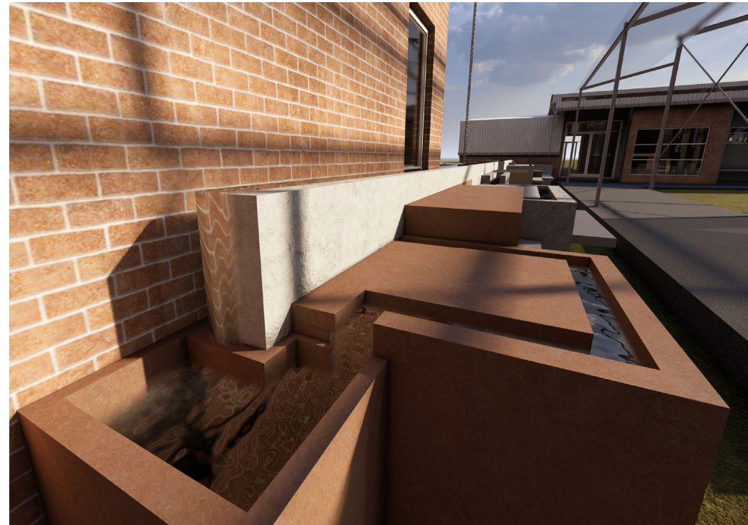
FIGURE 362:Water channels in the planter boxes at the resturant (Author, 2023).
