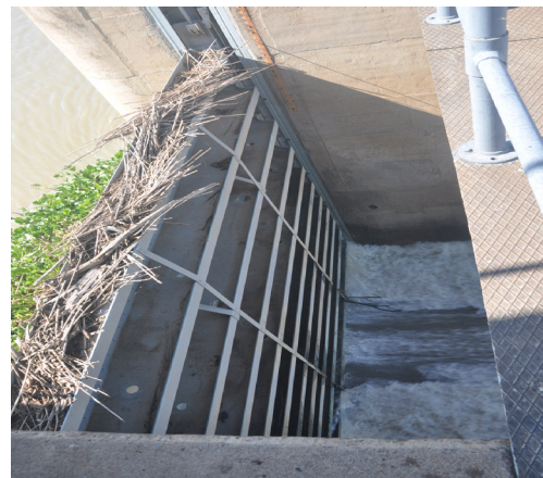
FIGURE 17: Sluice open to a minimum (Author, 2023).
