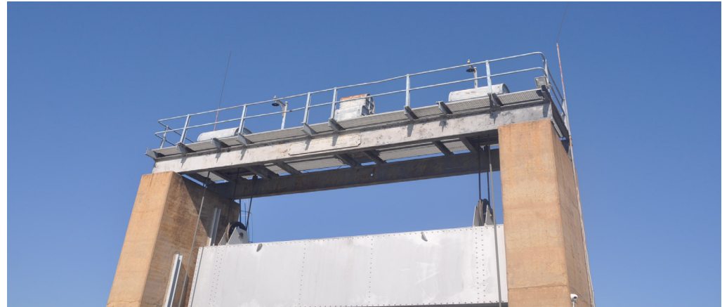
FIGURE 16: Counter weight system, controlling the sluices. (Author, 2023).
