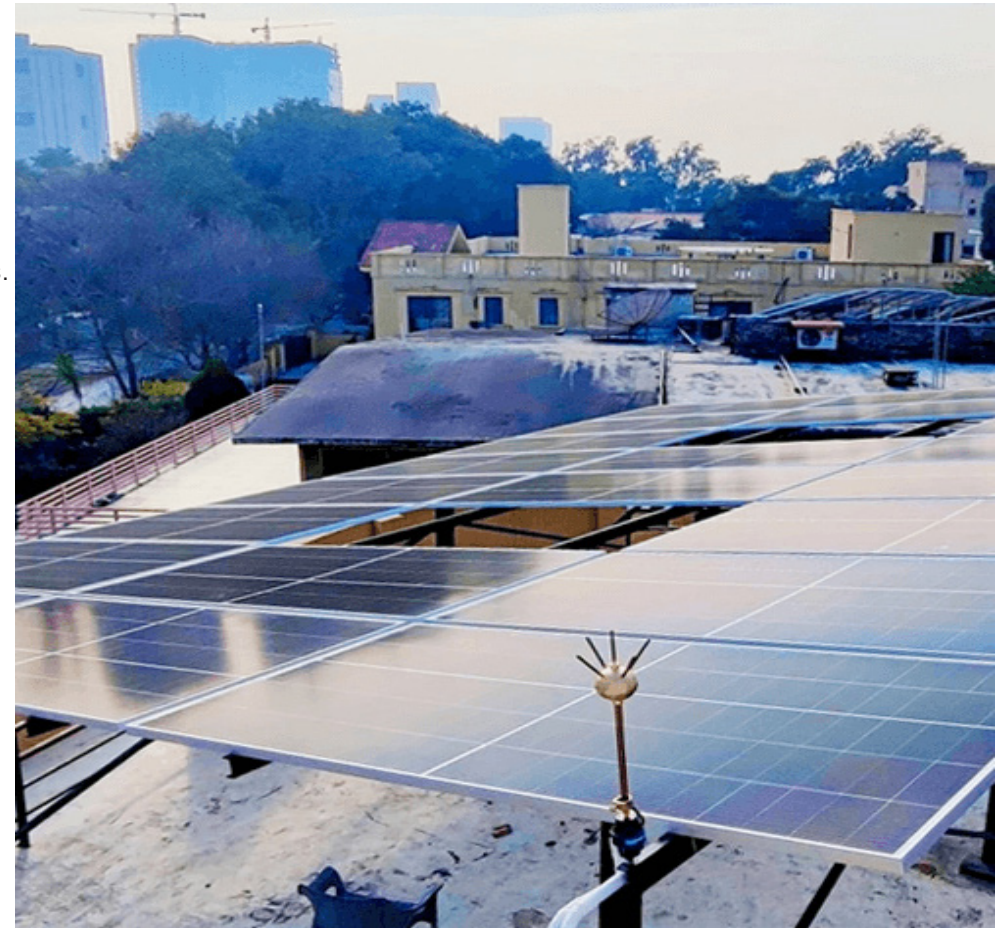
FIGURE 365: Ariel view of PV system (Wilson, 2023).
