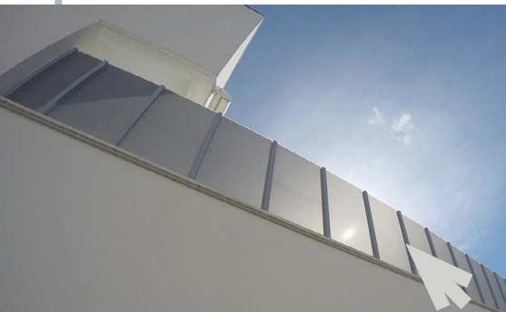
Figure 87 - Photovoltaic railings in a private residence located in Avila, Spain. (online www.onyxosolar.com )
