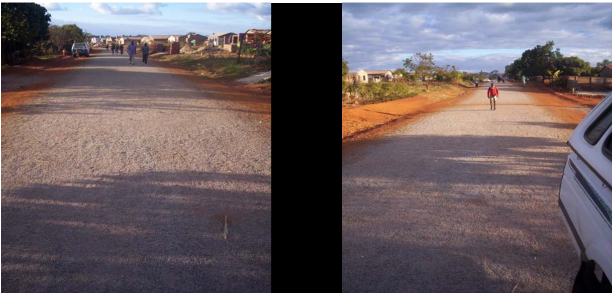
A consortium of cooperatives in Hatcliff are finishing constructing the access road using only their subscriptions
