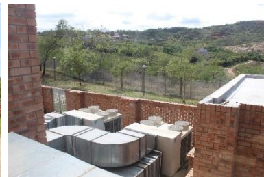
Generator and fuel room
