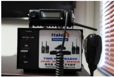
Emergency Communication Room / JOC
