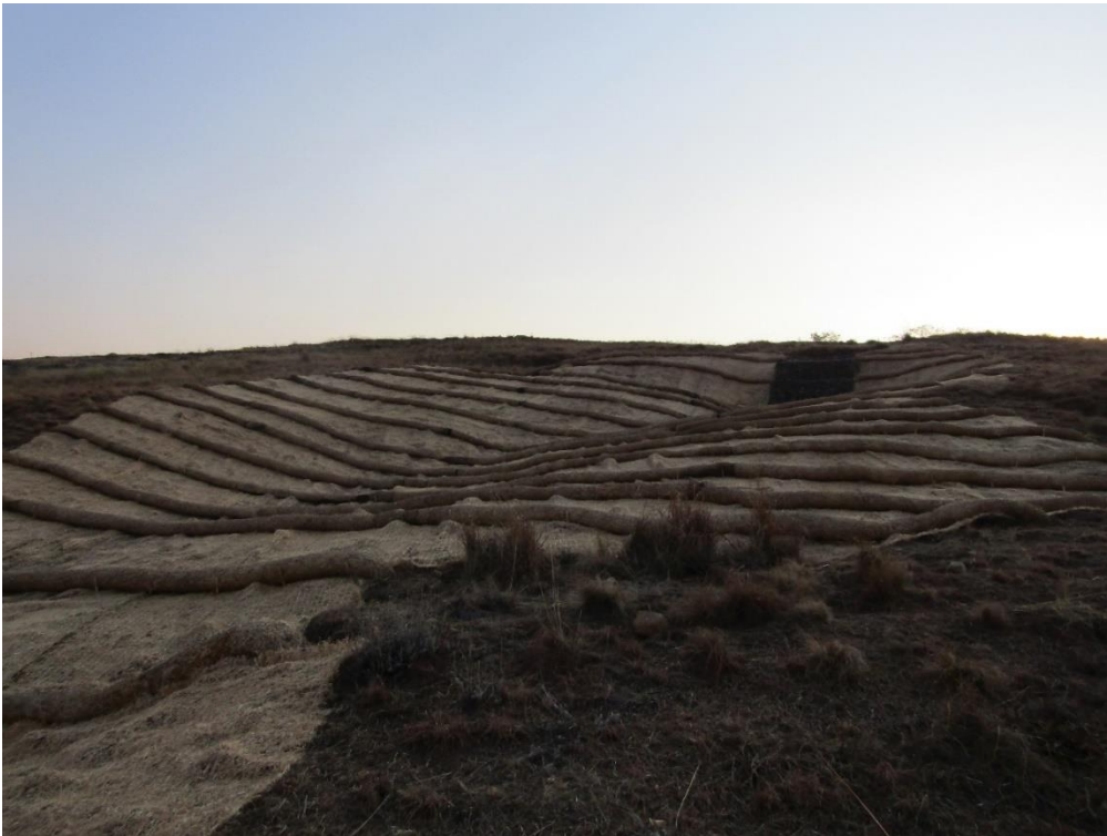
Fig. S5.1c: Newly rehabilitated site with new implements including erosion control blankets and fibre rolls placed over the displaced soils, taken in August 2018.
